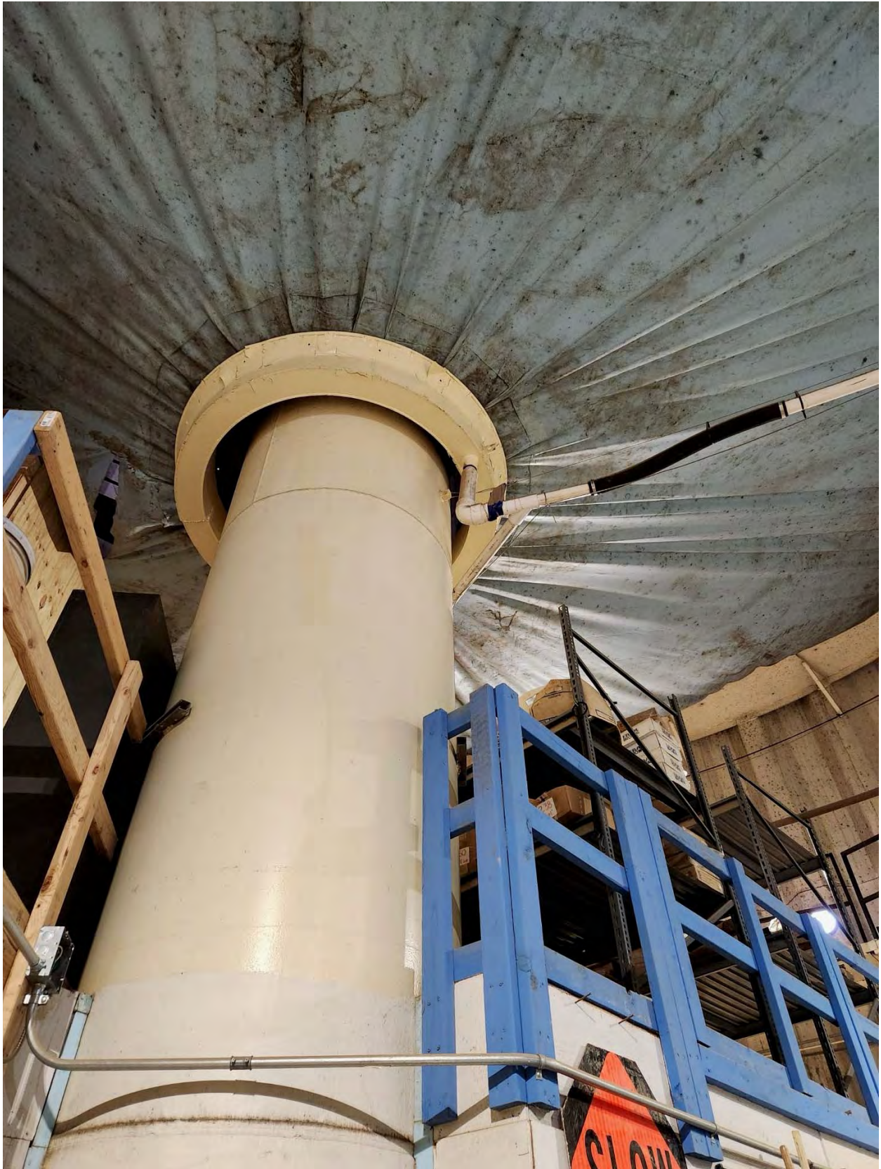
Photo 5 - Existing Interior Condensation Collection System and Interior Dry Wet Riser / Inlet/Outlet Pipe
