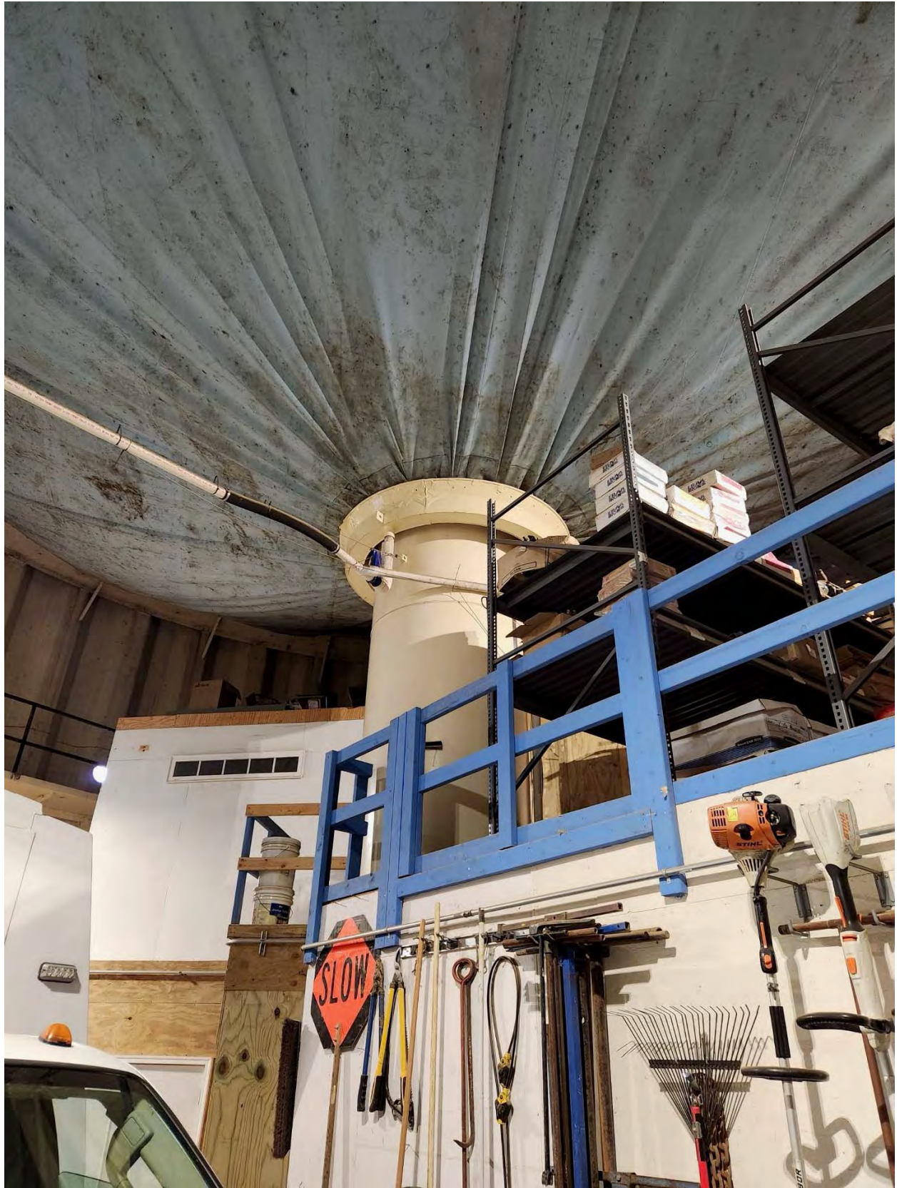
Photo 6 - Existing Interior Condensation Collection System and Interior Dry Wet Riser / Inlet/Outlet Pipe
